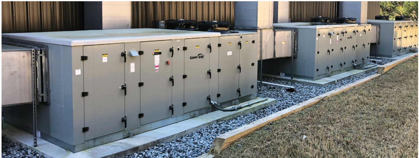
At the Alō Farms’ Peachtree City facility 3 packaged GrowAire™ dehumidification system units (@ 280,000 BTUH each) maintain 75°F and 55% relative humidity.
