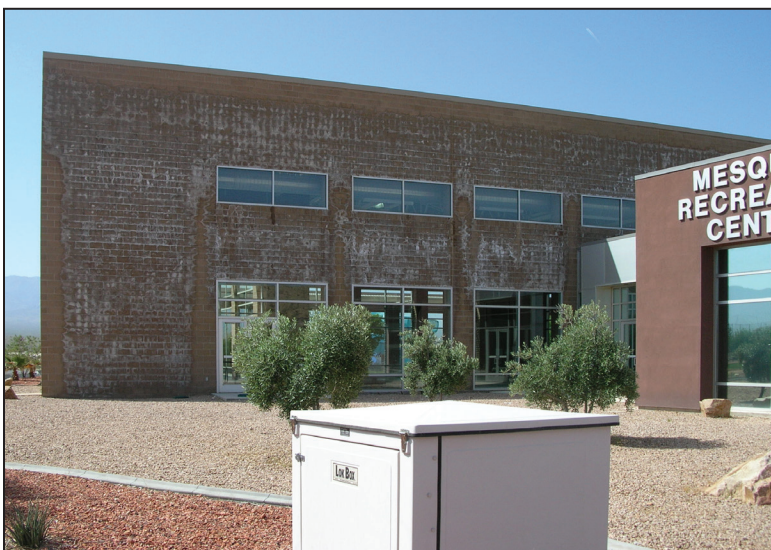
Figure 4. Example of natatorium without vapor barrier showing white chalking on building exterior
