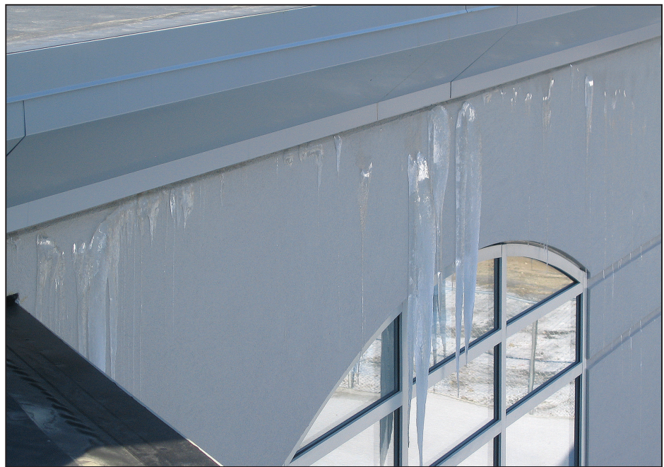
Figure 5. Example of natatorium with improper seals showing moisture migration and icicle formation
